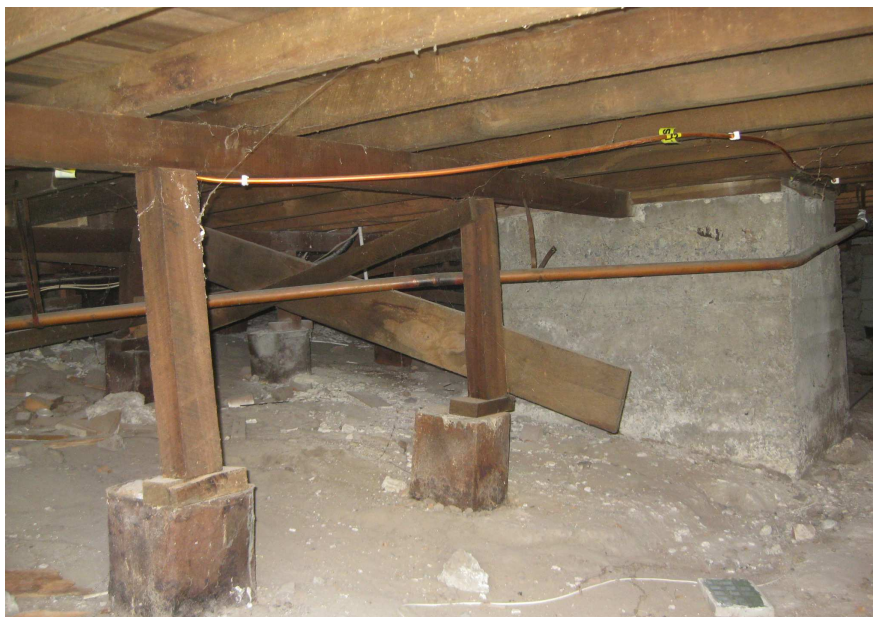
Figure 1: Jack studs beneath a hillside dwelling (tilt due to superstructure lateral displacement)
