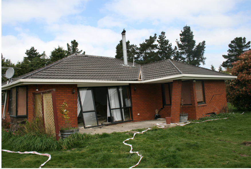
Figure 2: Severely damaged house from differential ground settlement and lateral spreading
