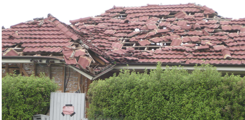
Figure 4: Dislodged concrete roof tiles
