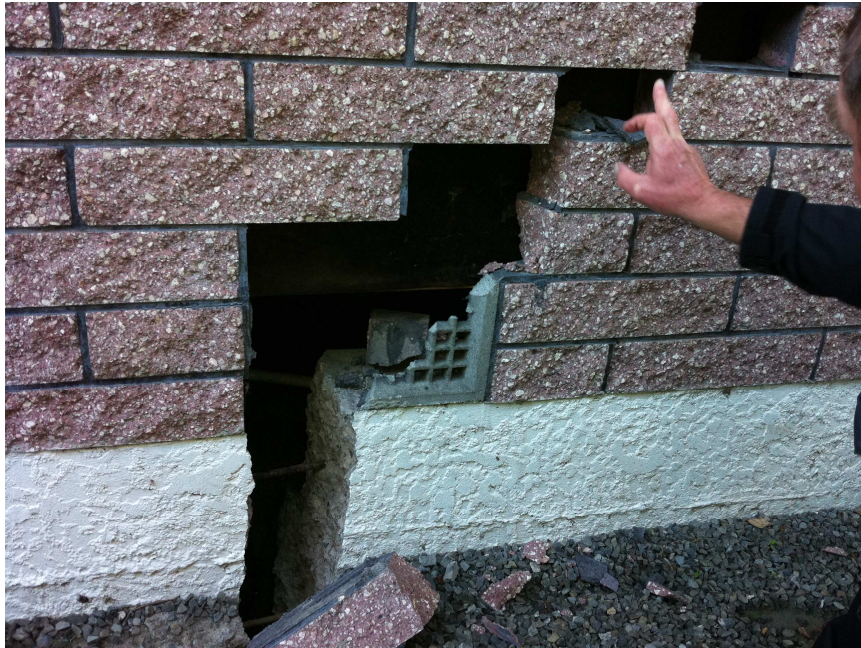
Figure 3. Example of reinforced concrete perimeter foundation pulled apart by spreading ground
