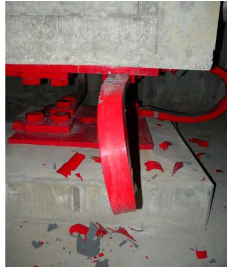
(b) Deformation of steel damper
