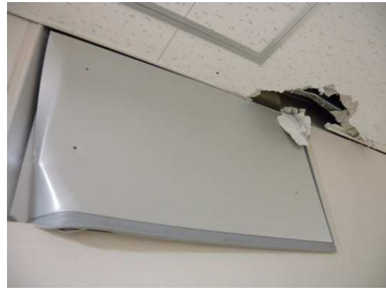
(b) Damage to the cover panel
