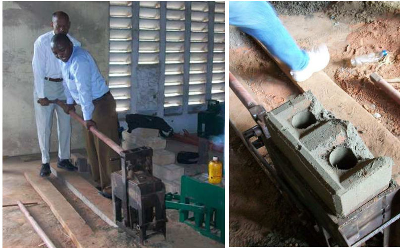
Figure 1: Manual compression of blocks and example of damage
