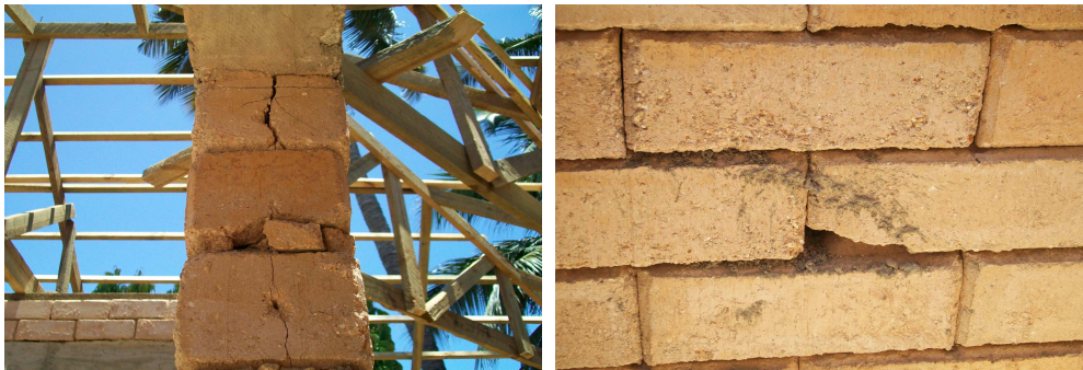
Figure 2: Cracking during construction
