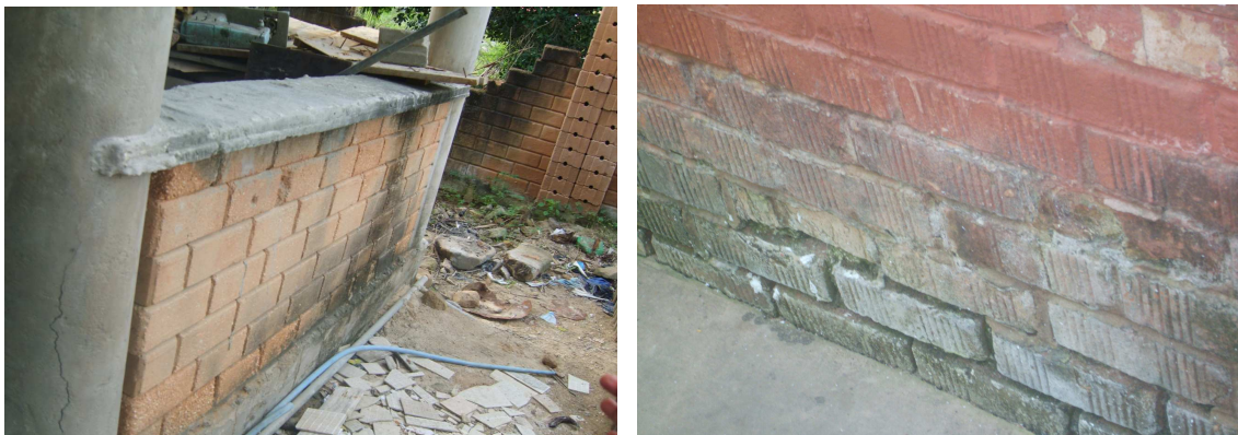
a) Efflorescence on a building that is still under construction
