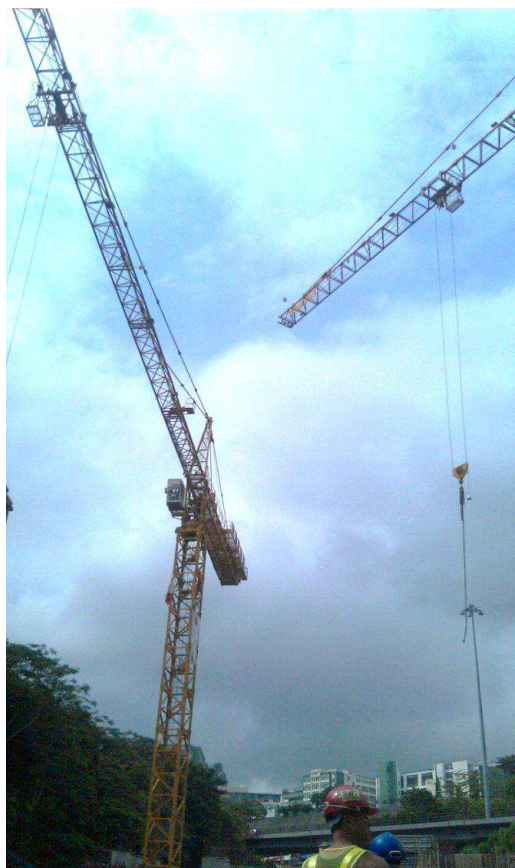
Figure 2. Tower Cranes in China with Collision Monitoring
