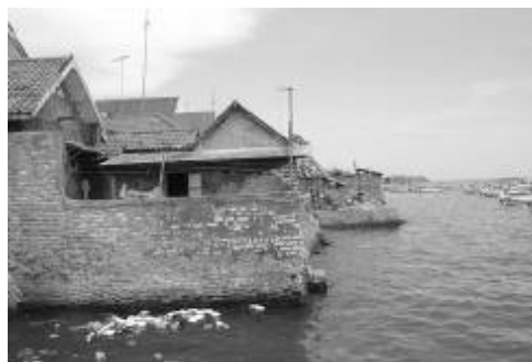
Figure 8: A protection wall against tidal waves that was built in different phases
