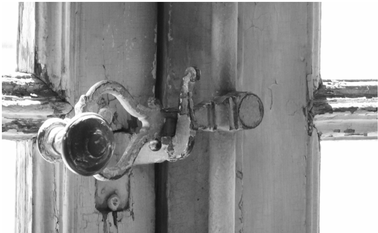
Figure 2. Details and Texture of old windows do not exist in modern windows: Original Window from 17th century, Dijon, France
