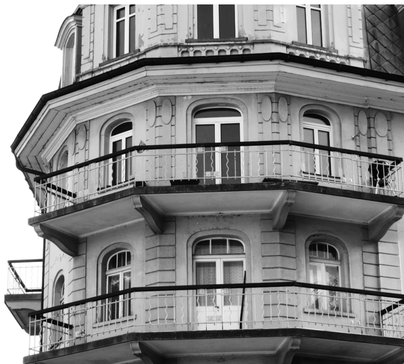
Figure 3. A residential building from beginning last century in Davos, Switzerland where the upper floors have changed to new windows, whereas the lower floor has maintained the original windows.
