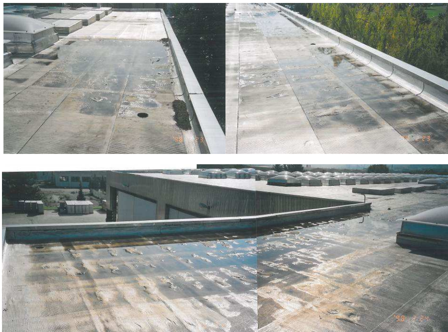
Pictures 6, 7 and 8: The water was unable to reach downpours, owing to deformation of the covering plane, and to limited slopes
