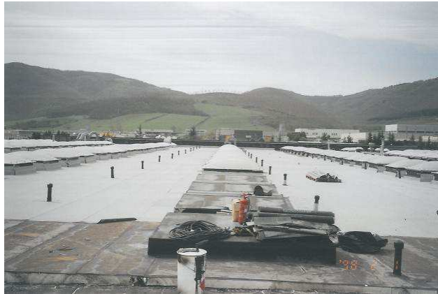
Picture 12: The lying of first layer of bituminous membrane was done partly, little by little was accomplished disposal of EPS panels for making slopes. You can see two coaxial roof vent, the one for venting original insulation, the second for evacuating possible condensations in EPS panels of slopes, and water that might enter during work
