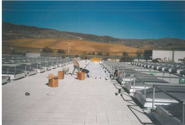
Picture 14: At the end, XPS panels (8 cm thick) of insulation were assembled and reinforced white concrete stones of floor, dry set on circular polypropylene bases, 2 cm high, for protecting and ventilating roof covering
