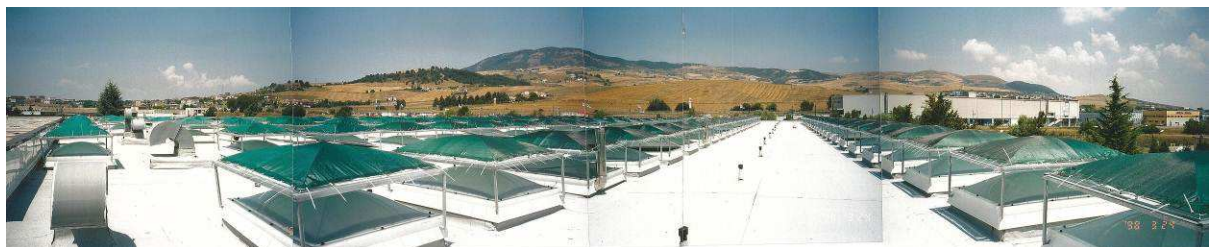
Picture 15: Then the insulations on the skylight and the flashings for protection and sunshades bases were assembled
