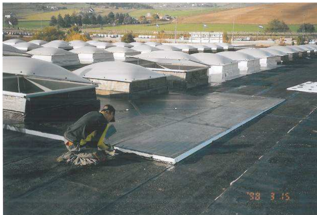
Picture 11: The assembling of new slopes, by means of cold gluing of more than 40% of surface, with bituminous & polymers based mastic . Panels were sealed on the perimeter, to avoid water penetration during work
