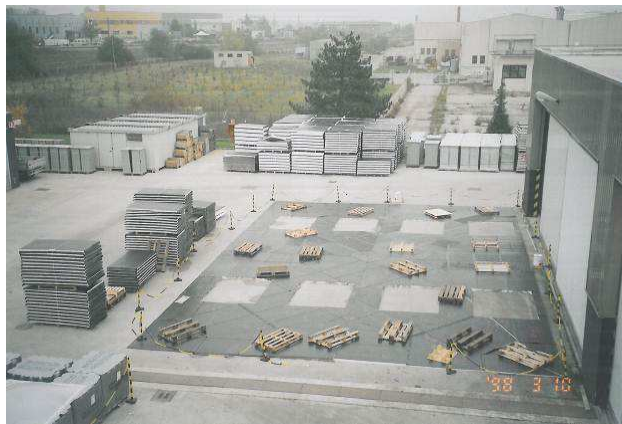
Picture 10: The tracing out, cutting, pre-assembling and numbering of the EPS panels with variable thickness for making slopes, has been made at the foot of the building, two spans in the same time, each of 18,00 x 12,00 m
