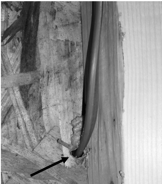
Figure 1: Poor Foam Air Sealing
