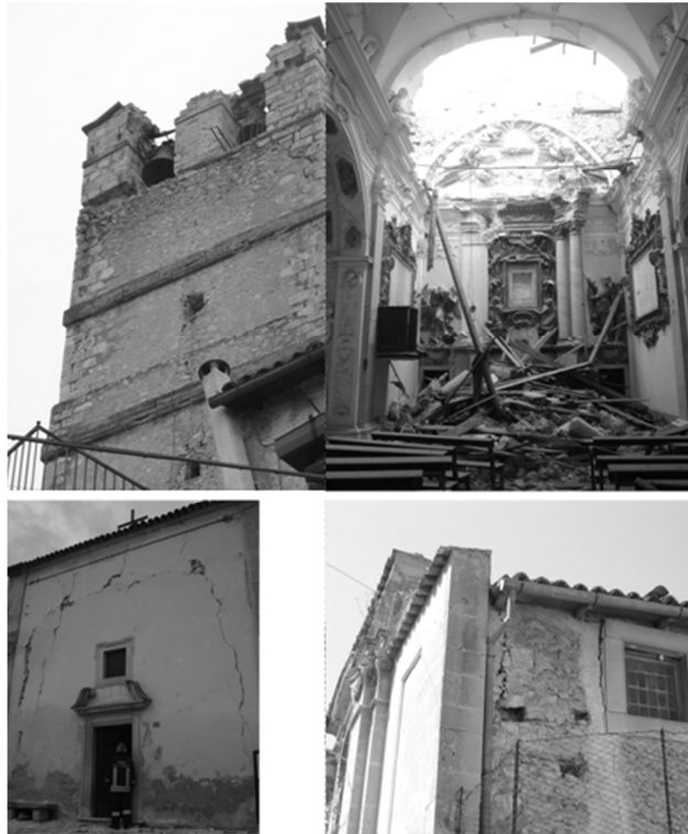
Figure 11. Example of damage suffered by the churches: starting from top left the churches of Santa Maria e San Vittorino (Carapelle Calvisio), San Marco Evangelista (Castel del Monte), Madonna del Rosario and Santa Maria del Carmine (Barisciano)
