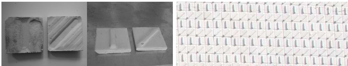
Figure 2: Building 15 – tiles details
