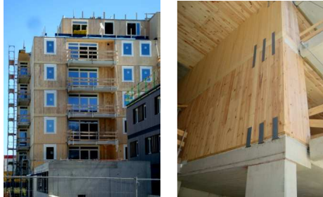
Figure 4 a and b: The Wagramerstrasse apartment complex, part of Vienna's 'Wood in the City' initiative, which now allows timber buildings up to 32 metres in height. Cores and ground floor podium are concrete. (Source: S. Lehmann, 2012).
